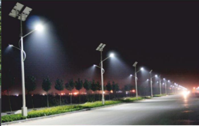
ROAD & STREET LIGHT
